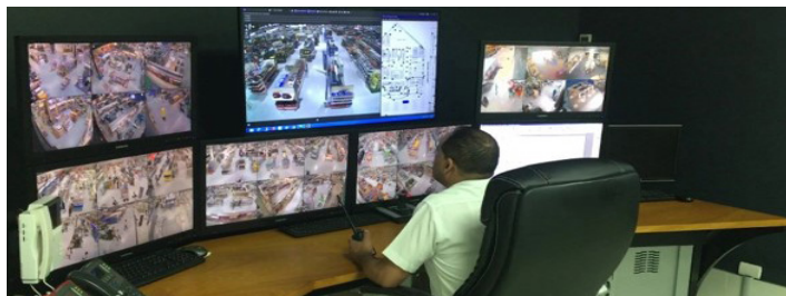
Ferreteria Ochoa central monitoring station
