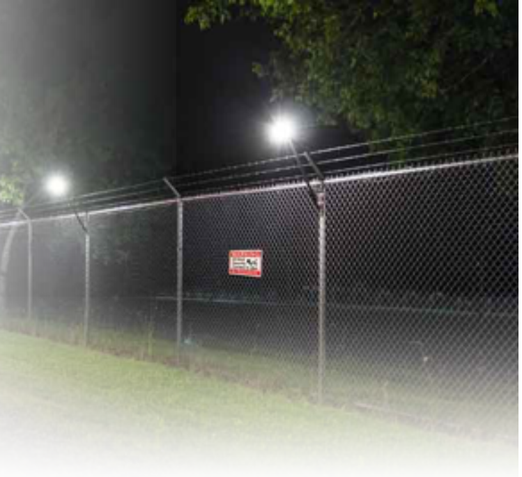
A site protected by a hybrid perimeter intrusion detection and intelligent lighting system
