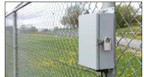
FlexZone processor on a fence
